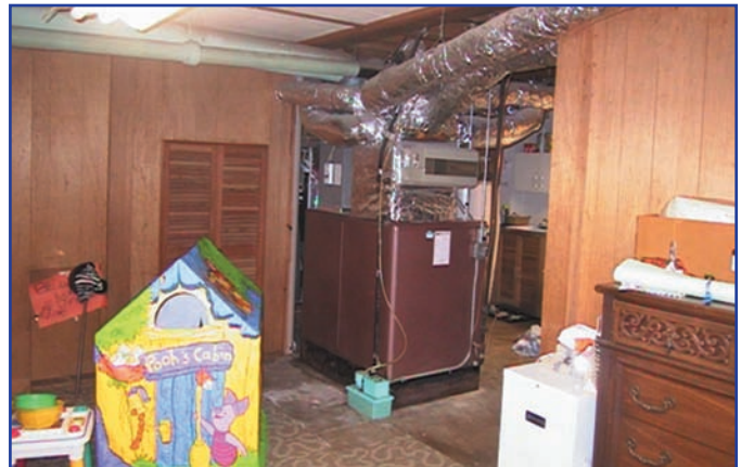
The original furnace and duct work in the house were circa 1970's. The air infiltration rate was 0.65 ACH (Air Changes per Hour) @ natural pressure. The ICYNENE LD-C-50™† application reduced the rate to 0.37 ACH nat .
