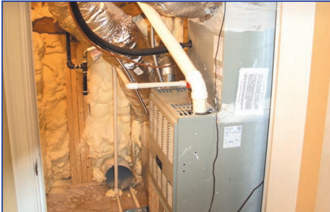
Icynene was sprayed directly into the wall cavity around the HVAC system and the return and supply ducts. This helped to improve the airtightness of the building envelope and increase the overall energy efficiency.
