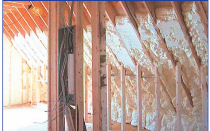
Icynene was applied to the underside of the vaulted ceiling in the old attic space. This turned the previously unconditioned space into a conditioned living area.
